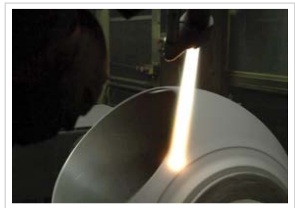
Protective coating being applied to ball valve to combat corrosion and wear.
